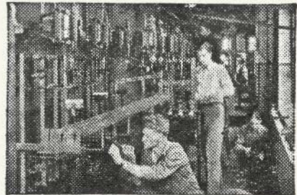
A Real Switchboard in the Coyne Shops
